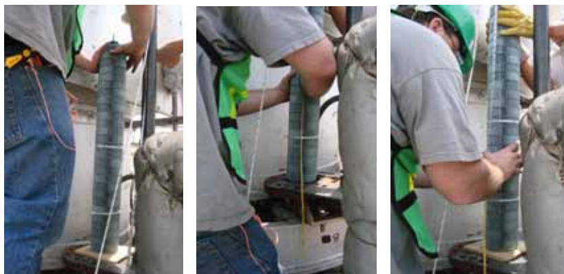
Figures 2,3,4 – The easy install was completed in two days by plant staff supervised by Catacel.
