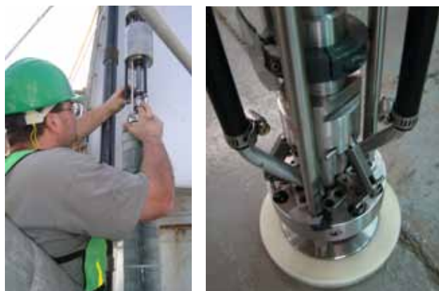
Figure 6 – Installation of SSR catalyst was done in 3-ft. long sections with tools designed by Catacel by sliding the media down from the tube top.
